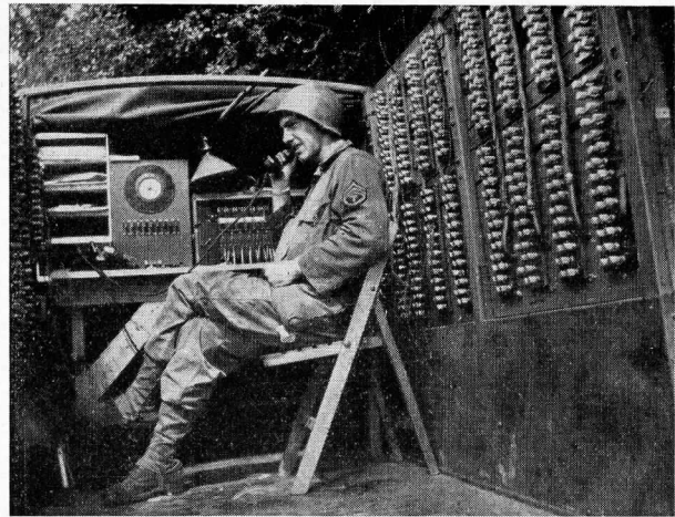
INTERIOR VIEW OF TRAILER AT LAVAL SHOWING TERMINAL STRIPS FOR CROSS-CONNECTING CIRCUITS AND DESK ARRANGEMENT.
