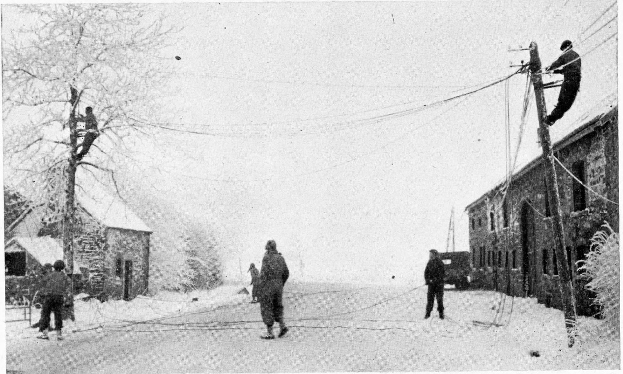
THESE MEN OF THE 35TH SIGNAL CONSTRUCTION BATTALION ARE SALVAGING WIRE IN BELGIUM (THIS PICTURE WAS TAKEN EARLY IN JANUARY).
