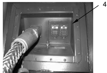
Containerized Latrine Power Panel 1000-Watt Floodlight Connections
