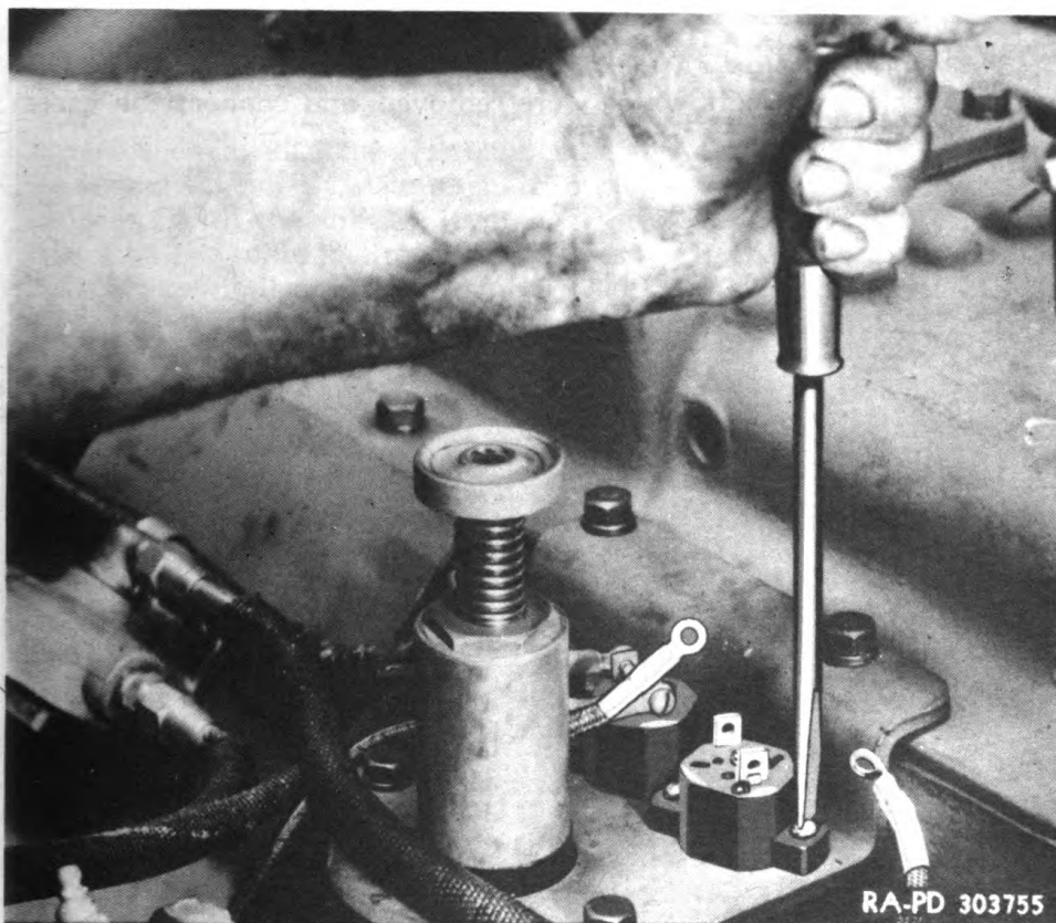
Figure 94—Removing Circuit Breaker
