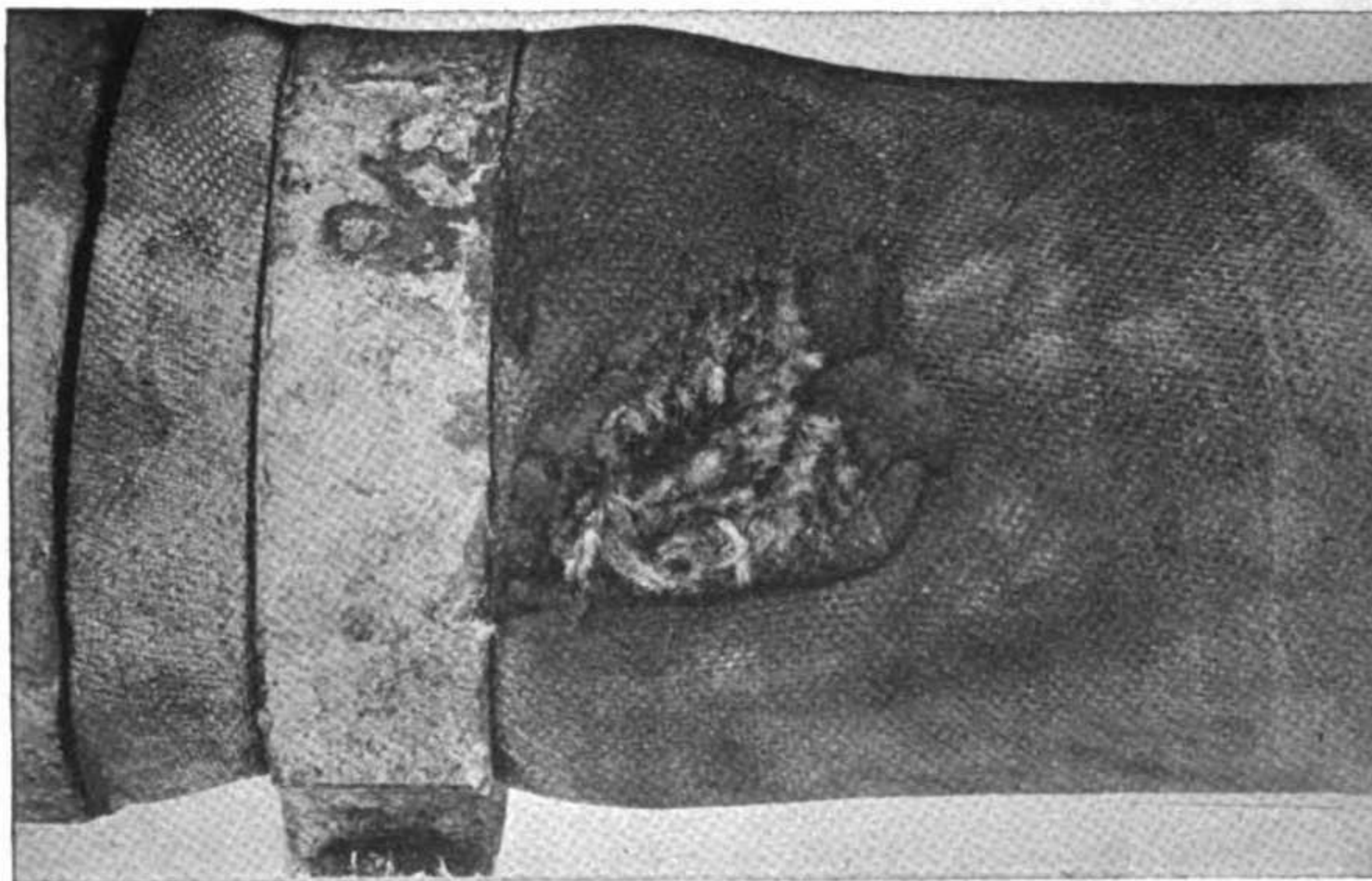
Figure 2. Hose with hole in outer cover and fabric at hole torn. When fabric at hole is torn or rotten, hose will be removed from service.
