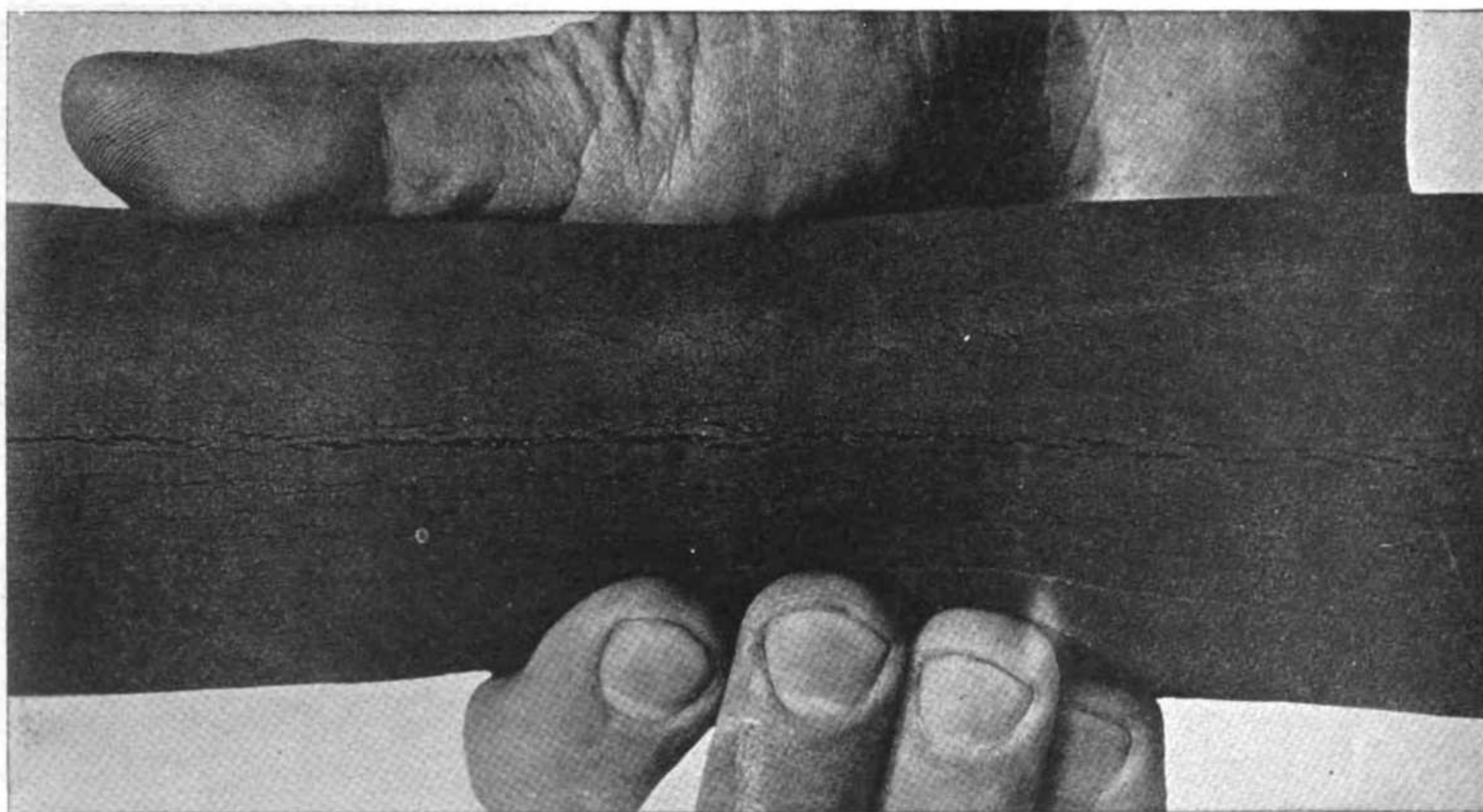
Figure 4. Hose with slight longitudinal crack. The crack in this hose is not serious enough to justify removal of the hose.
